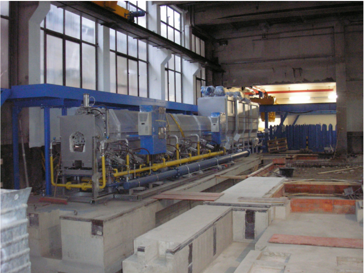
New block heater
